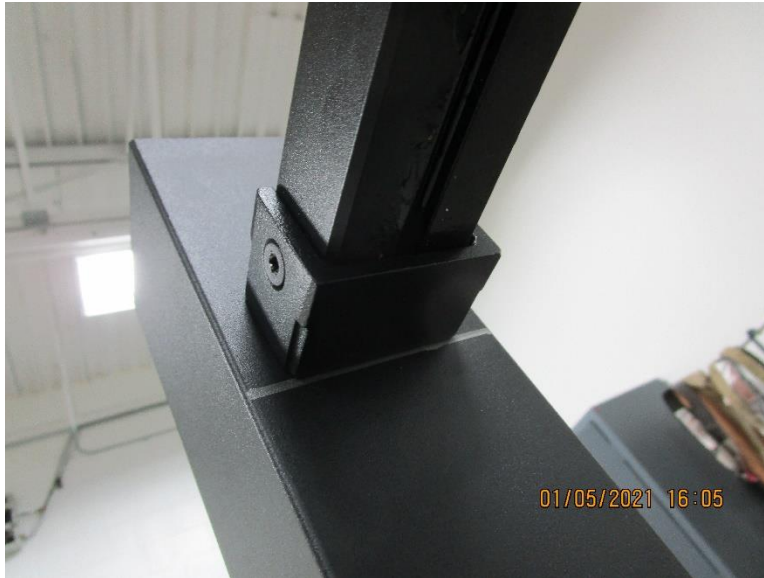
Photo No. 11 Bracket to Rail to Post Attachment
