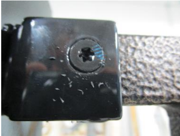
Photo No. 3 Bracket Attachment to Steel Post Mount
